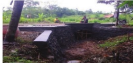
Talud Goron-gorong RT. 11 - 2017
